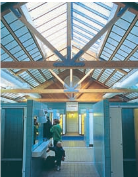
Avoid false ceilings in changing rooms. Use roof-lights to give a sense of space.
